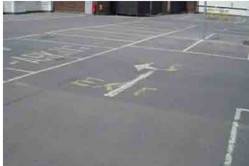
Figure 2-C Conflicting Signage in Tesco section of Car Park
